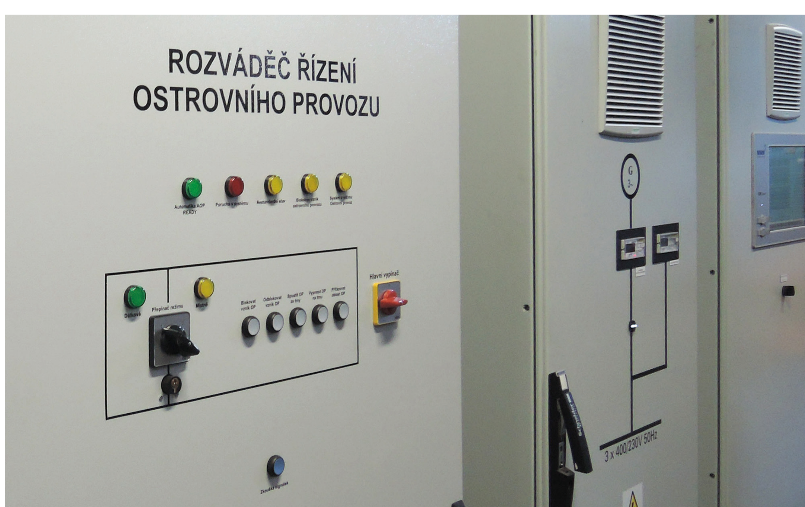
CHP unit and island operation technology control system
